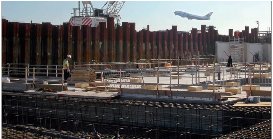
Steely determination: Keeping construction of the steel reinforcement of T2’s concrete sleeves on track was paramount
